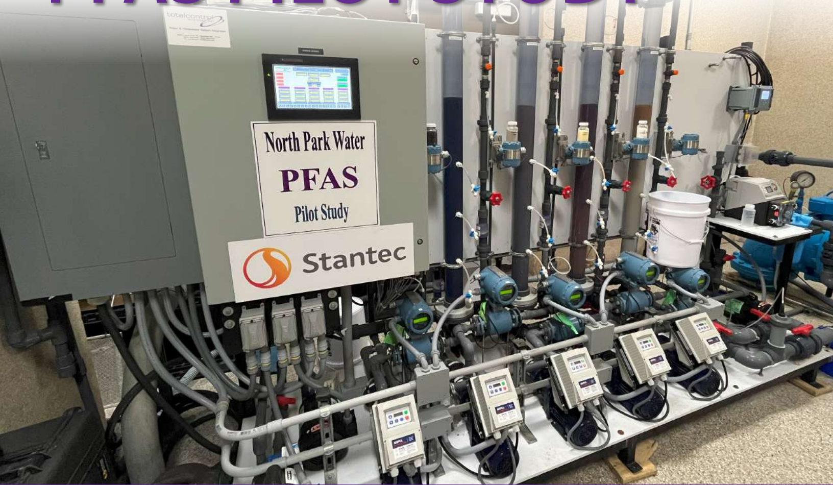
Figure 2. PFAS Pilot system built and provided by Stantec.
